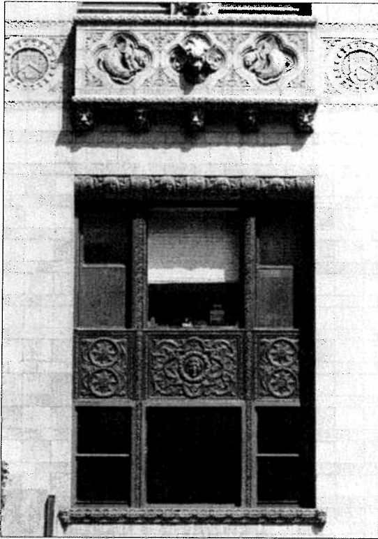
Left: Detail showing balconette at 4th floor and highly decorated windows of the 2nd and 3rd floor bank offices.
